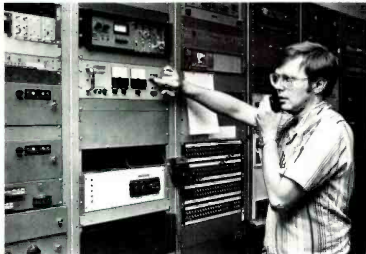
WKOW technician Jim Buntrock lines up microwave receiver by SMR with news van in the field.
